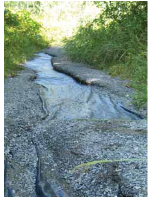
The Great Meadow Loop, part of the Village Connector Trail system, experienced erosion to a lesser extent
