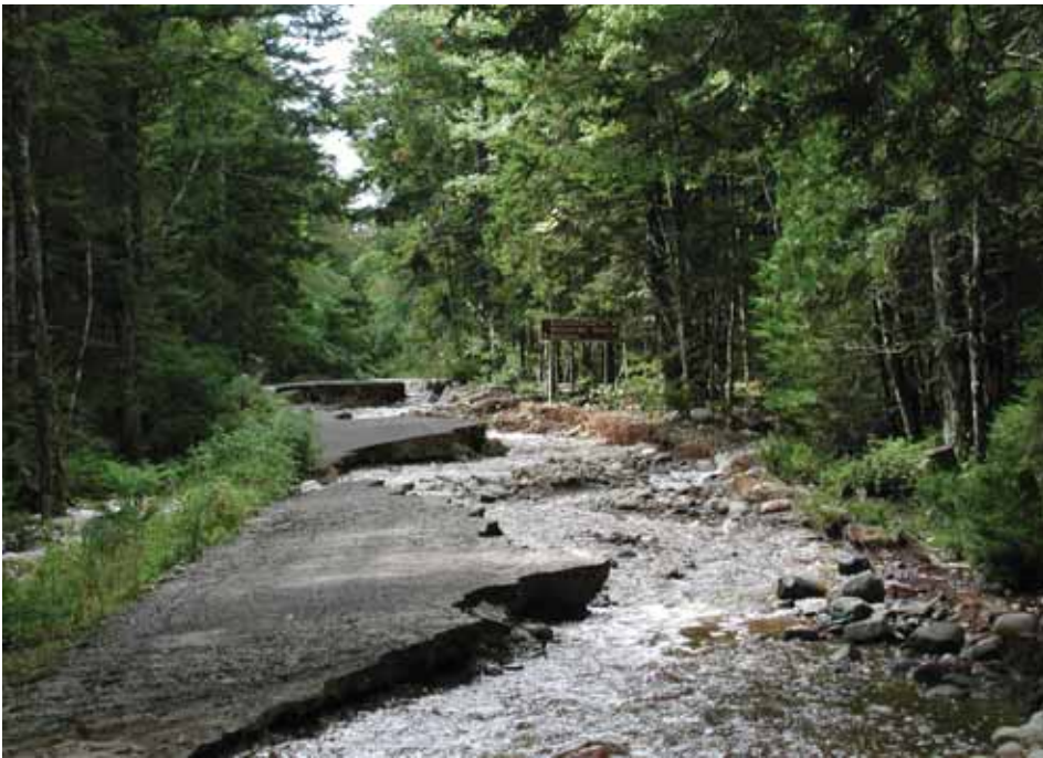
The Seal Cove Road, shown here, suffered severe washouts in 2008 due to Hurricane Hanna.
