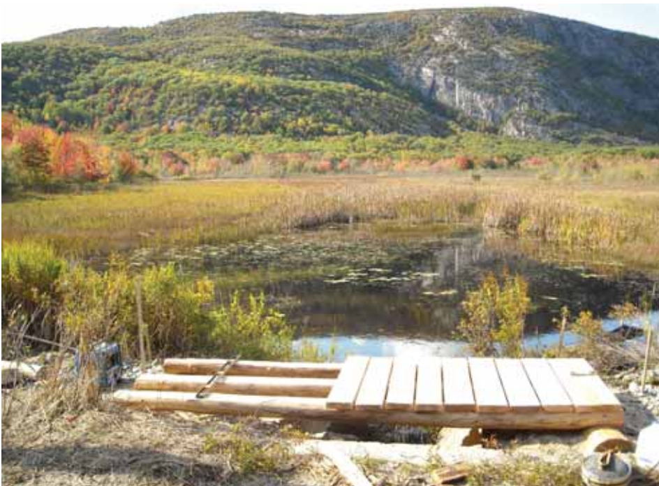
An in-progress look at Jeff’s Bridge, at site 3 on the Schooner Head Path.
